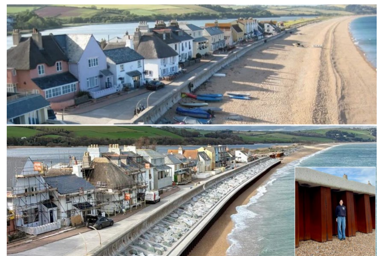
Fig 6. Beach levels in early January 2026 were around the top of the pile cap ie slightly lower than shown in the top picture. Bottom picture, and inset, show levels in early February 2026 – the lowest on record. (credit: Start Bay Inn Facebook)
